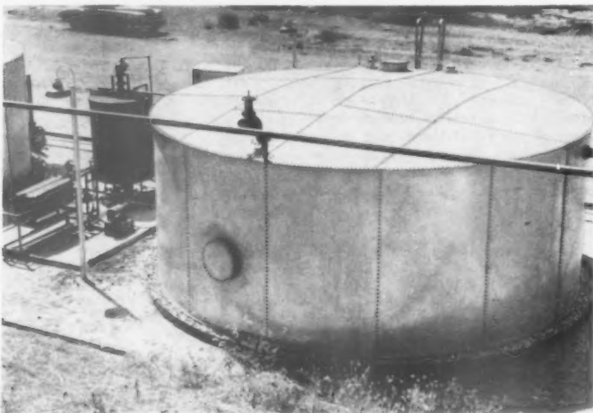
SUNRAY OIL CORP. uses this closed-system, diatomaceous earth filtering plant in Newhall-Potrero field. It has a brine output of only 350 bbl. daily, but the company was required to inject it underground.
